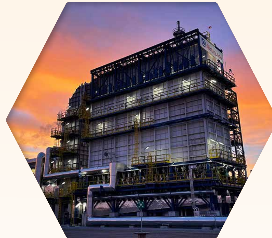
Air Liquide and Covestro launched a new-generation hydrogen production unit
