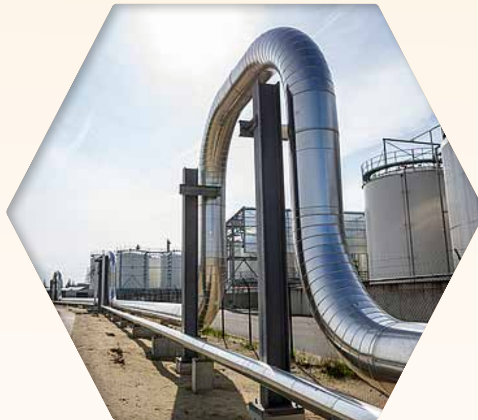
Europe's biggest industrial heat network ECLUSE connects several chemical companies
