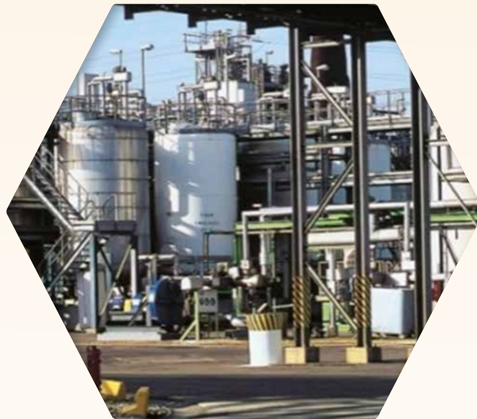
Plastics2Chemicals: Pilot installation Indaver to convert end-of-life plastics into chemicals
